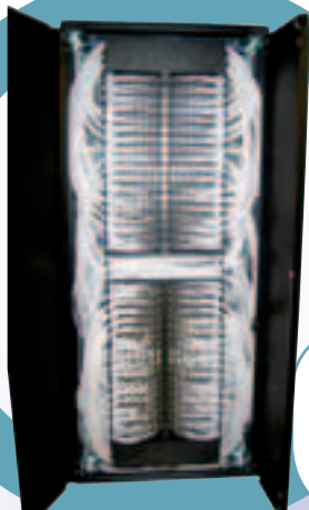
High Density Copper Cabling Cabinet page 20
